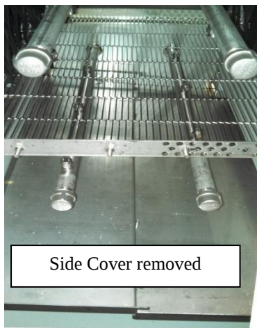
Figure 4: Pre-Wash Containment with Side Cover Removed
