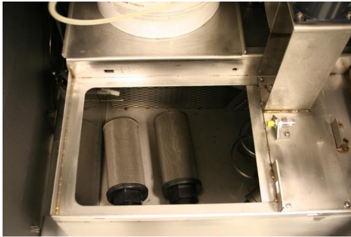
Figure 13: Batch Intake Strainers
